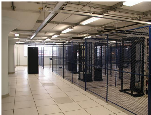
Fire Rated Partitioning
